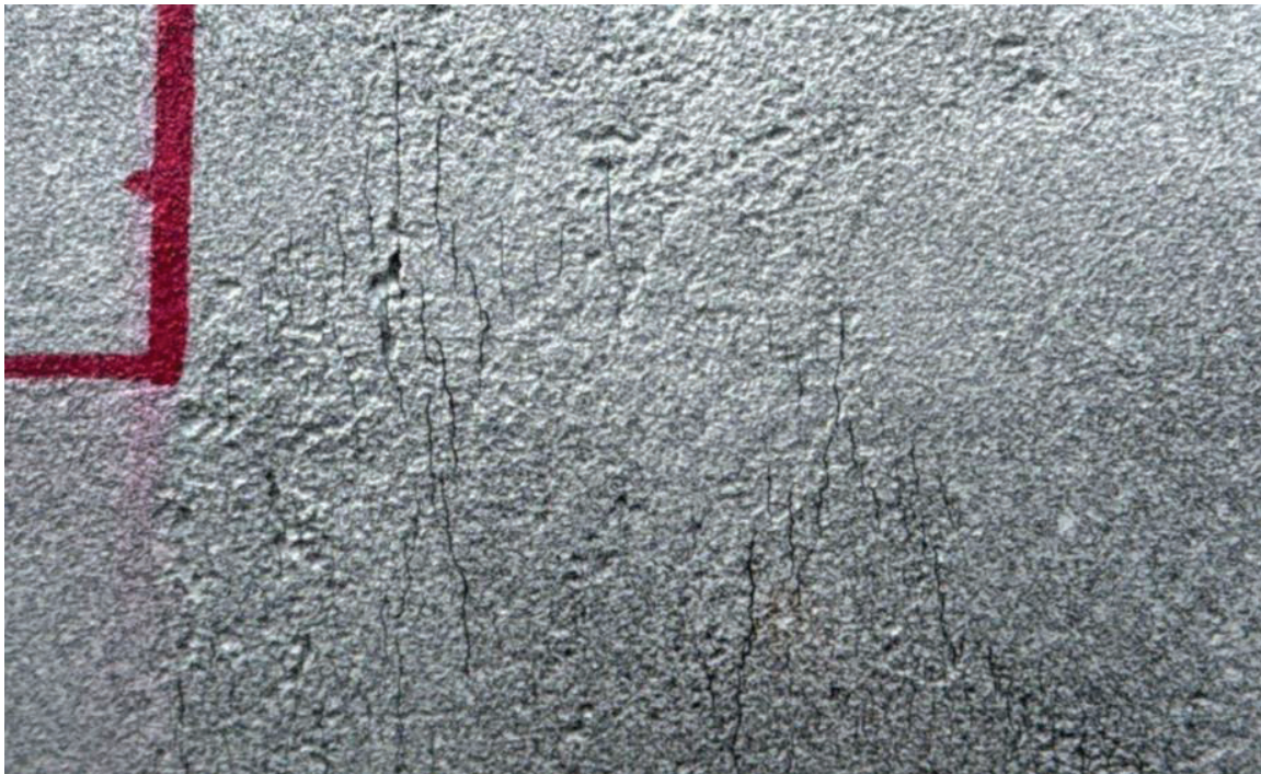
Figure 8: As-found CSCC anomalies for the ILI data shown in Figure 6.
