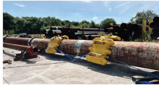
Figure 8: Unsupported pipe under bending due to 4 tonne static weight
