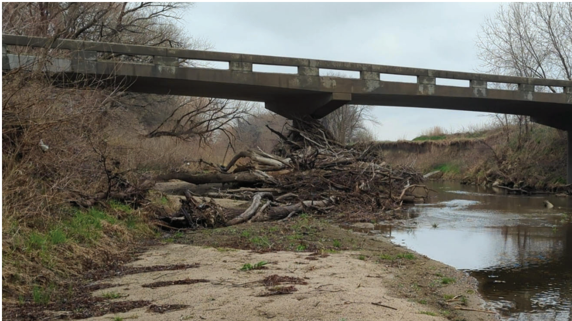
Figure 4. Debris Obstruction on West Pier of Upstream Bridge
