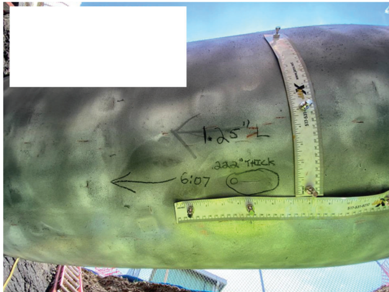
Figure 10: DNT-2 with metal loss and crack
