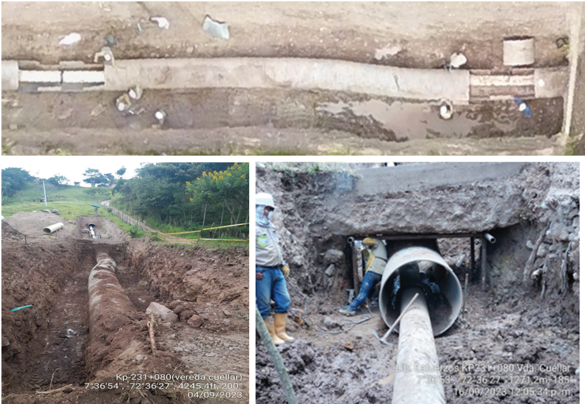
Figure 12. Downstream flank of the movement showing pipeline displacement and eccentric casing section view. (Source: CENIT)
