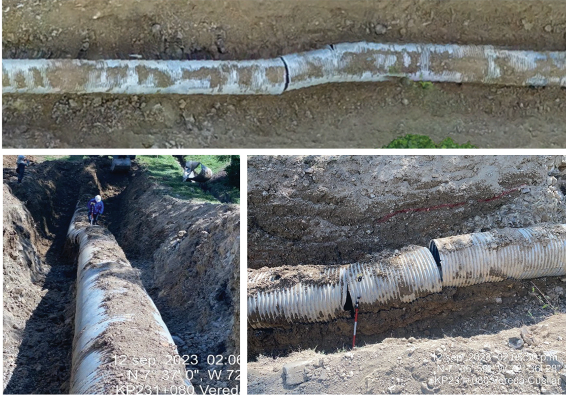
Figure 11. Upstream flank of the movement showing displacement and fracture of the external casing. (Source: CENIT)
