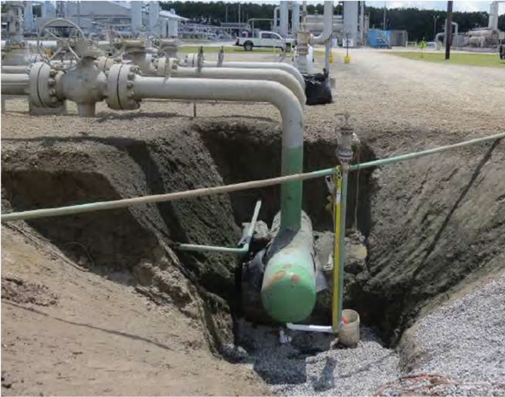
Figure 5. Example of Header Dead Leg and Low Point Drain excavated for leak repair. [12]
