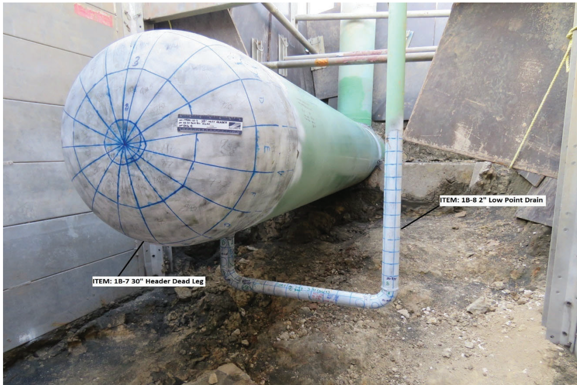
Figure 7. Example of the same Header Dead Leg and Low Point Drain in Figure 6. [12]
