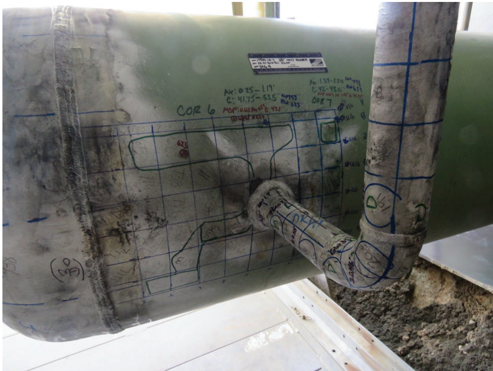
Figure 6. Example of Header Dead Leg and Low Point Drain excavated for inspection. [12]
