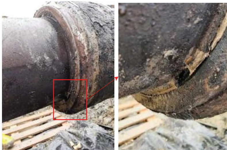
Figure 5. Corrosion micro-vent detected by the Vibroacoustic Technology upon reactivation of a pipeline
