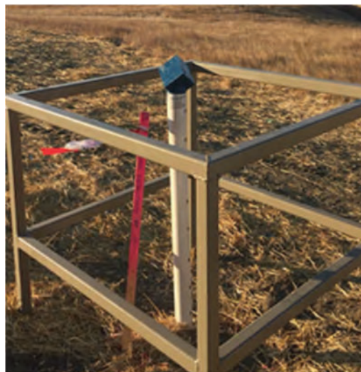
Fig. 1: SubSense monitoring an underground transition point of a buried pipeline
