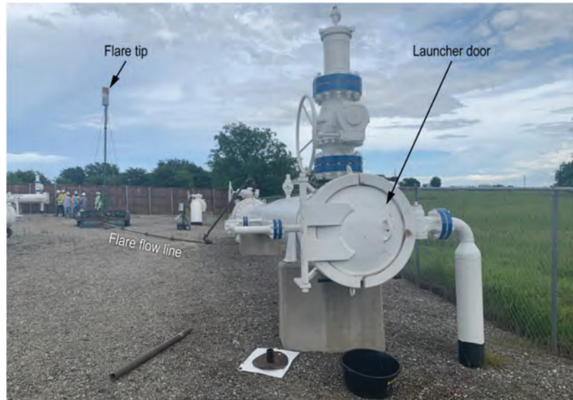
Figure 1. Pig launcher and flare tip at accident location near Farmersville, Texas
