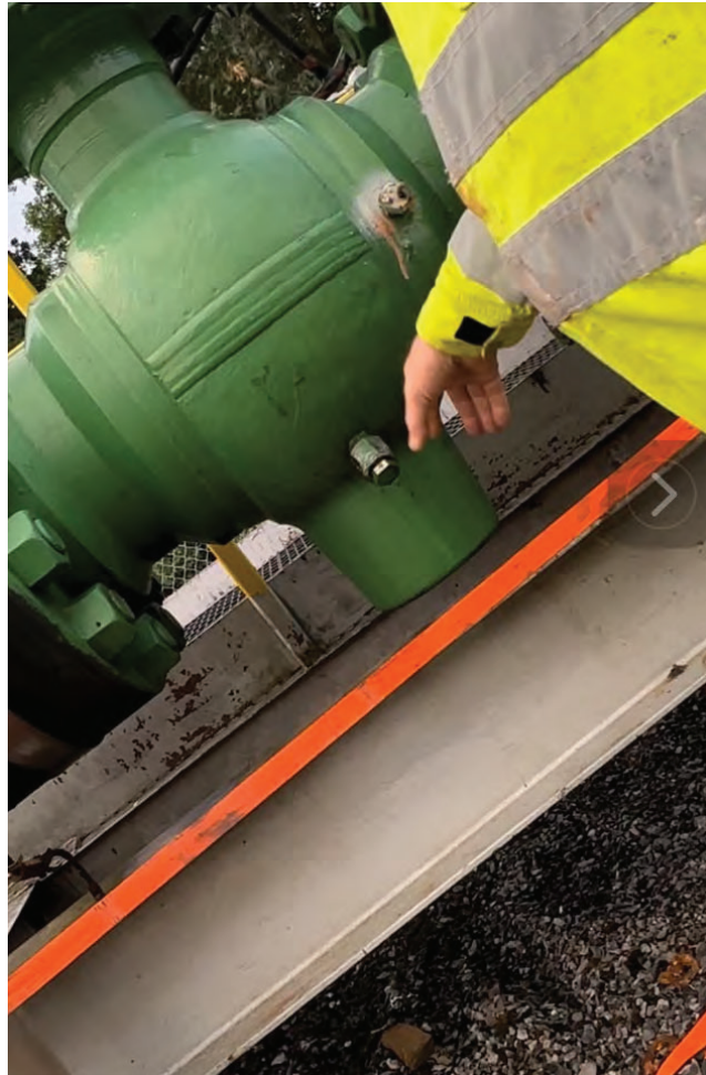
Figure 7. Bleeding valve used to alleviate pressure due to a valve leakage
