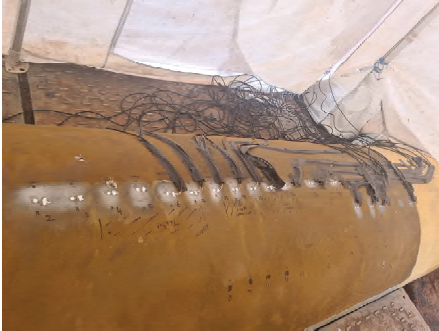
Figure 3. Strain gauges installed at site
