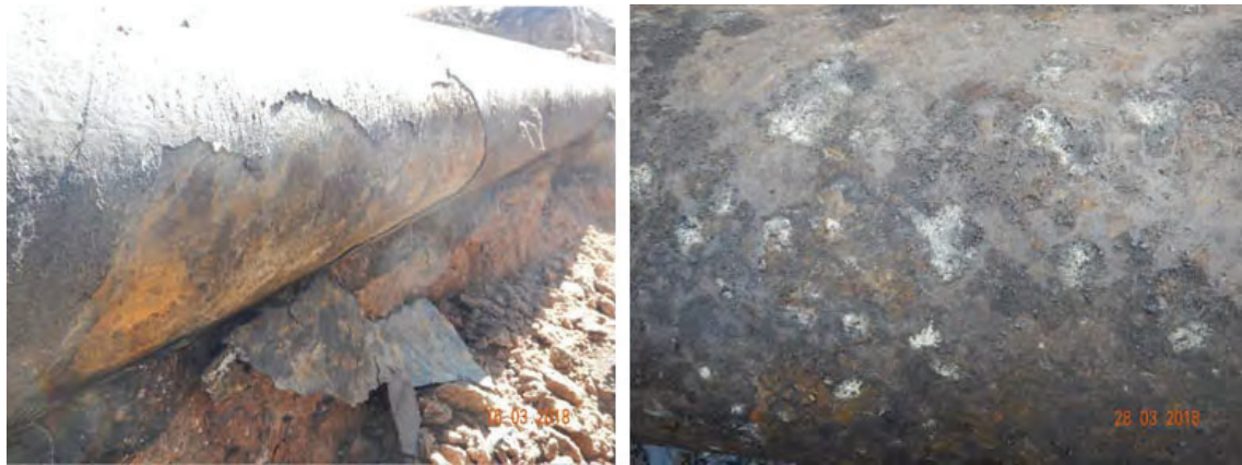
Figure 1: Coating condition and whitish deposits found in excavations
