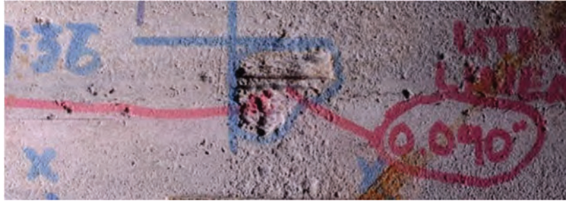
Figure 1: Confirmed SSWC in ERW pipe material
