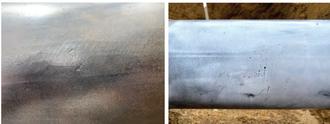
Figure 16. Corrosion Feature at 15182.347 m. Longer length reported by ILI appears to be due to the corrosion defect being, mostly, ground out during construction.
