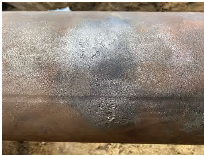
Figure 15. Corrosion feature at 9248.145 m.
