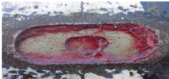
Figure 14a: Defect within defect
