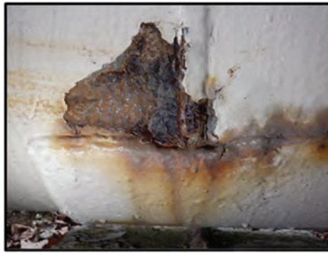
Figure 4. Typical external corrosion example: crevice corrosion.
