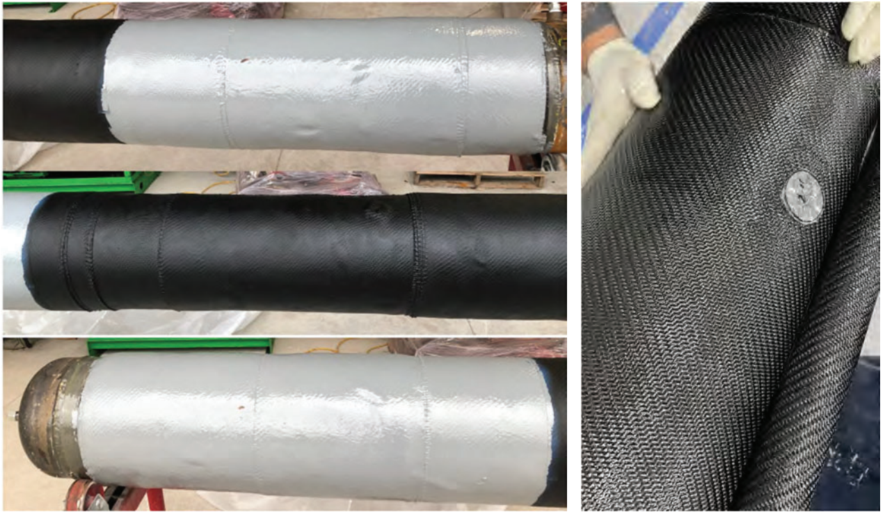
Figure 2. 10-in sample before burst test with composite repair with air pocket defects
