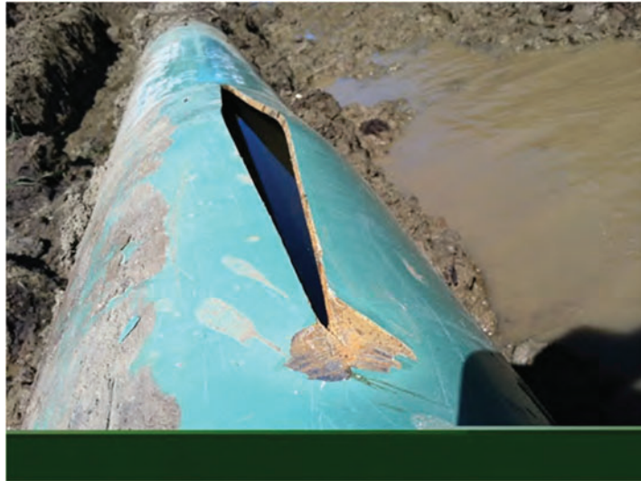
Figure 1. Case 1 - Seam failure of 2012 installed pipe during hydrostatic test
