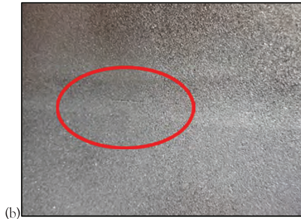
Figure 4(a-b). Case 4 - Lack of Fusion Long Seam failure of 2019 installed pipe
