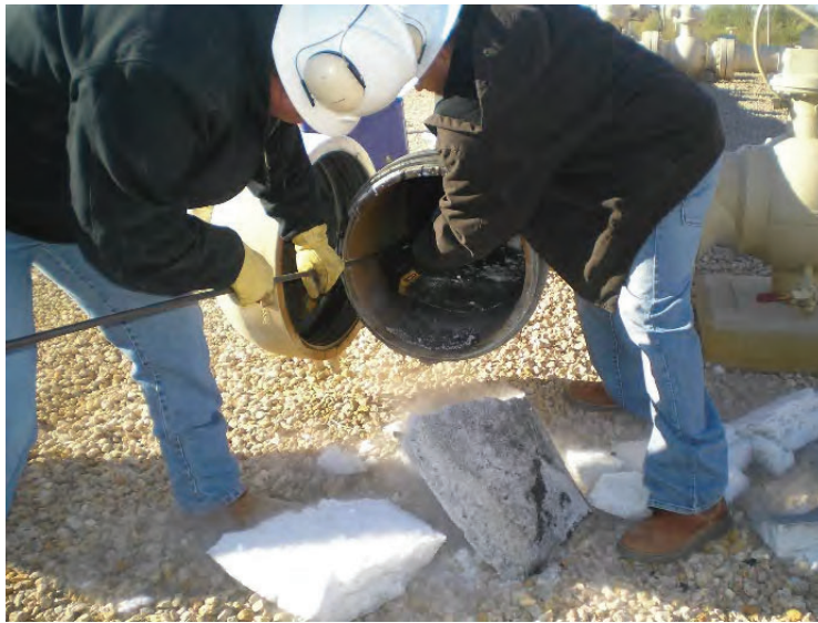
Figure 4. Removing a Cleaning Tool from a Carbon Dioxide Pipeline (Presence of Dry Ice)
