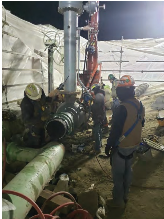
Figure 10. Isolation of a Carbon Dioxide Pipeline
