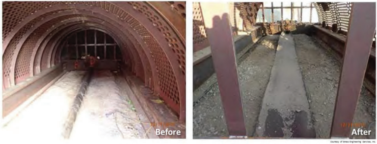
Figure 1. Photographs showing the post-test response of a running fracture.
