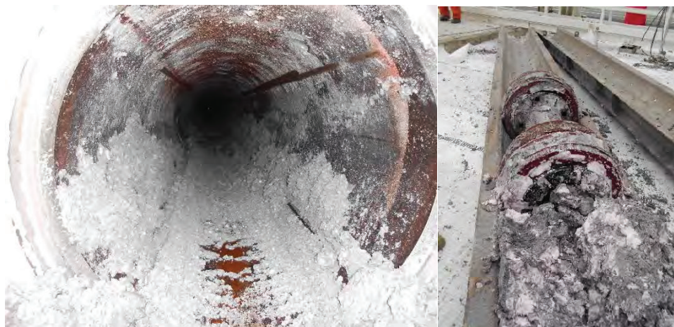
Figure 1-2. Examples of previously removed debris.
