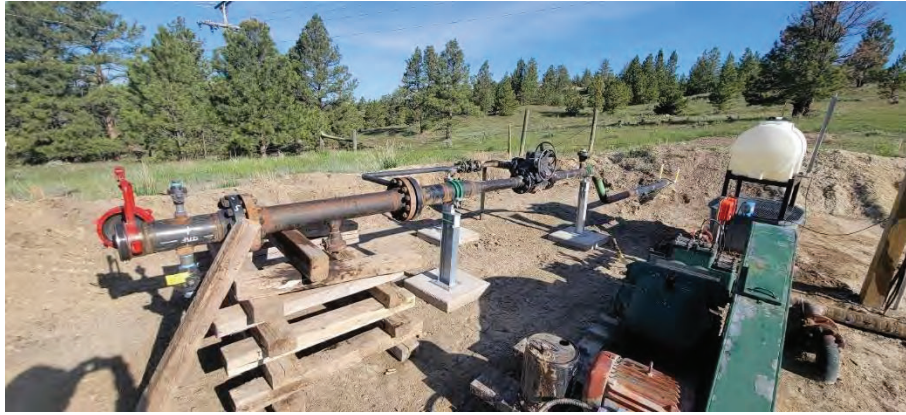
Figure 18. Launcher area, noting low spot as pipeline goes uphill after the launch.
