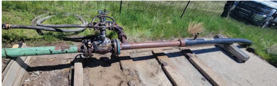
Figure 16. Receiver where the 4" pipe comes out of the abandoned 6" pipe.
