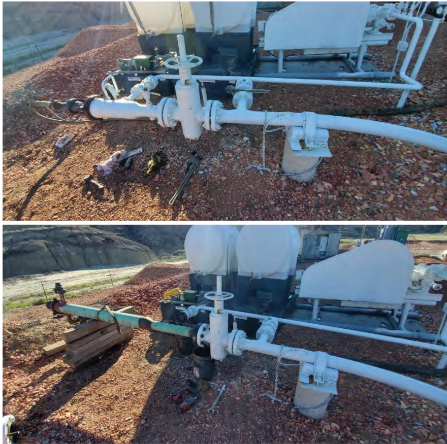
Figure 3. Trap before and after extension.
