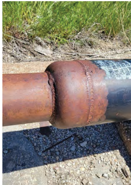
Figure 17. Closeup of where the 4" line emerges from inside the 6".
