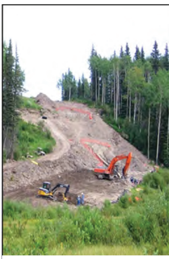
Figure 4a Landslide movement parallel to pipeline
