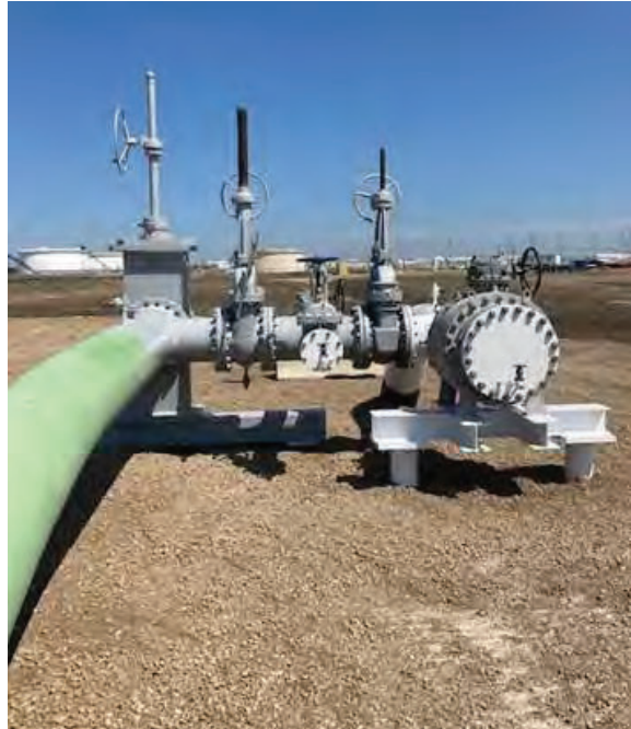
Figure 7. Topping valve and entrance point
