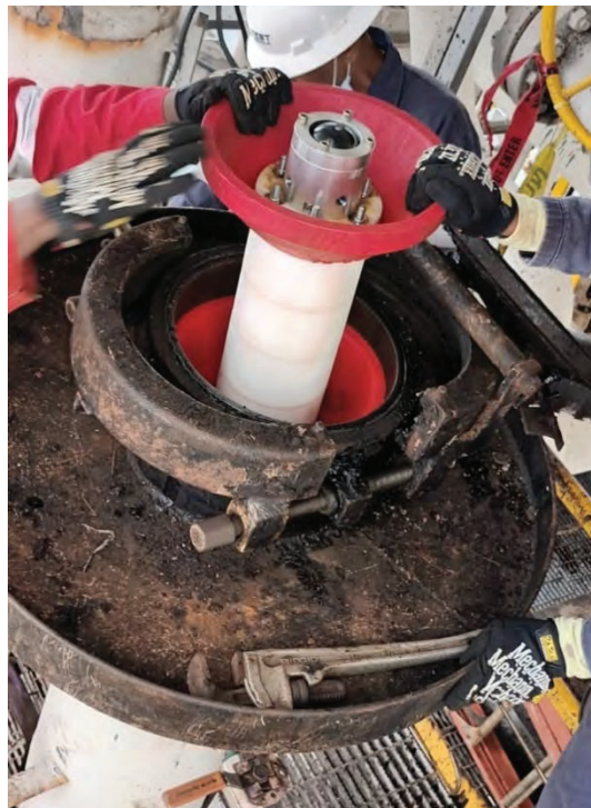
Figure 2: Maintenance pig integrated with a Multi Sensor Inspection Ball (Chevron South Africa Strategic Business Unit)
