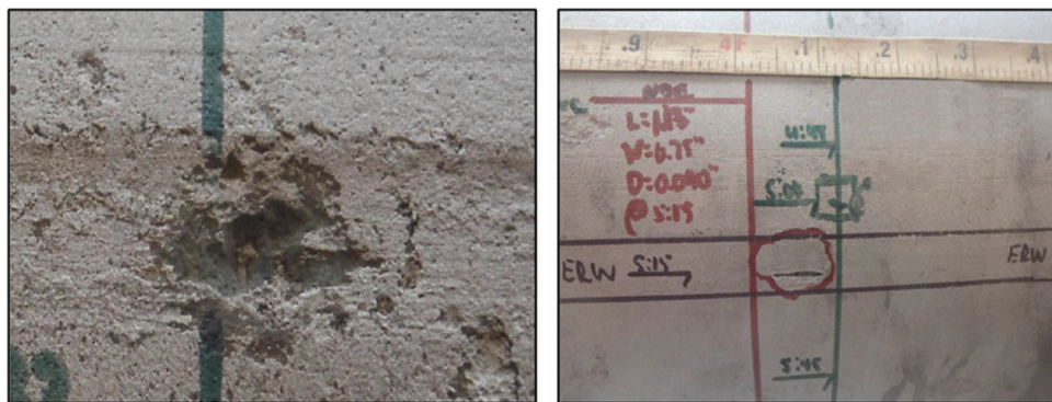
Figure 10: Examples of features investigated based on SSWC classification model results with general corrosion (left) and preferential (right).
