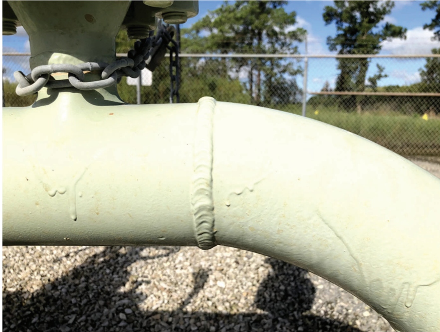
Figure 5- Location of 3.6” restriction in -schedule 80 bend and tee. Also note the high/low weld.
