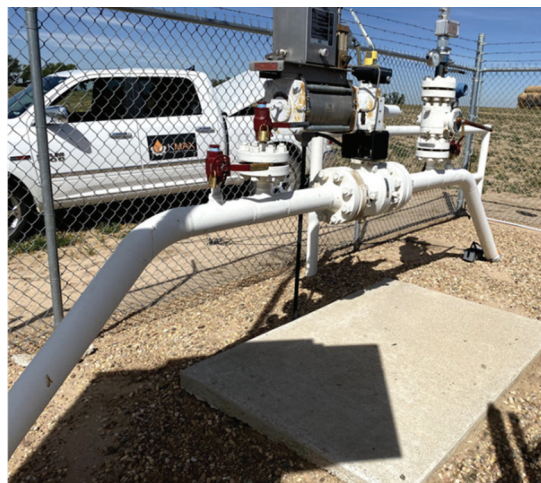
Figure 7. Above ground valve setting with heavy wall tees
