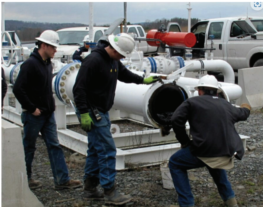
Figure 4. Technicians' proximity to pipeline traps.
