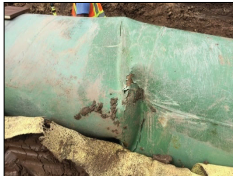
Figure 1: Illustration of pipeline failure and buckling
