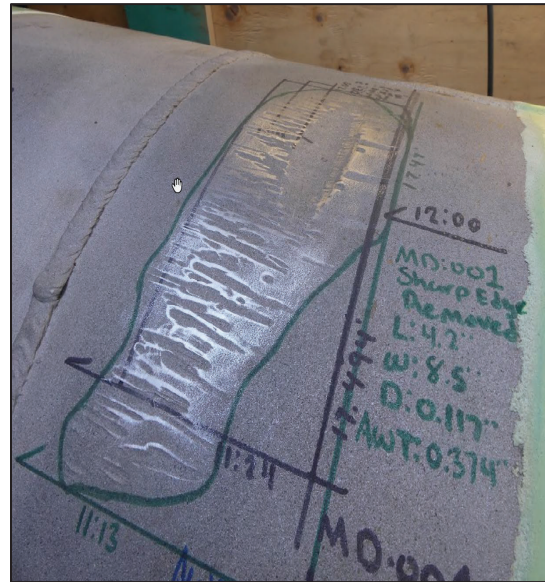
Figure 4. Defect area no stress risers.
