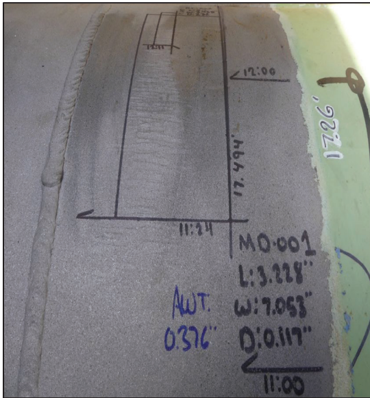
Figure 3. Defect area with stress risers.
