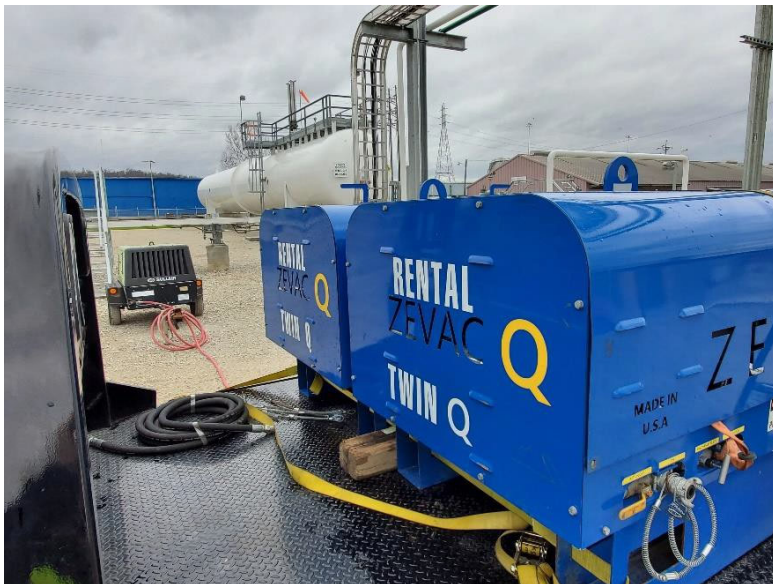
Truck-mounted ZEVAC unit in operation.
