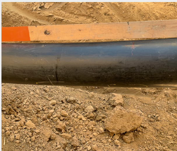
Figure 7: Pipe bend in the vicinity of the defect (at the red cross).
