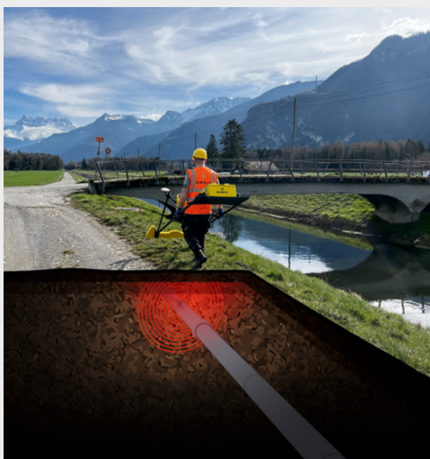
Figure 8: Hand-held CMI detector in use. The red circular lines around the pipe illustrate the magnetic field generated by the signal generator.
