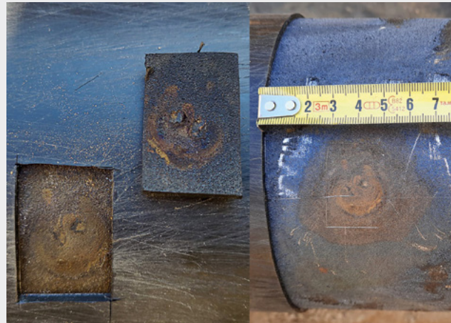
Figure 6: Defects identified with CMI. Left: Excised 3LPE coating. Right: Close-up of the defect with the disbonded area.
