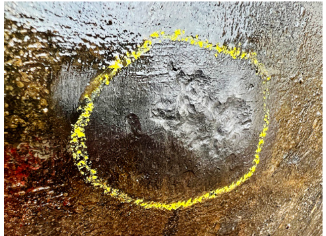
Figure 2: Verified anomaly, ext. corrosion at 3 o'clock, at a coating defect
