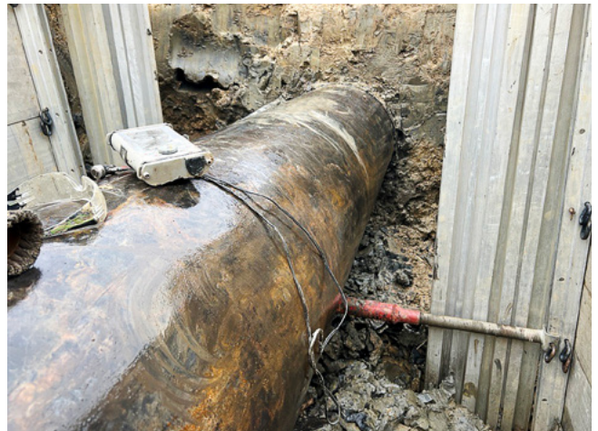
Figure 3: Exposure of internal anomaly, int. corrosion at 5 o'clock
