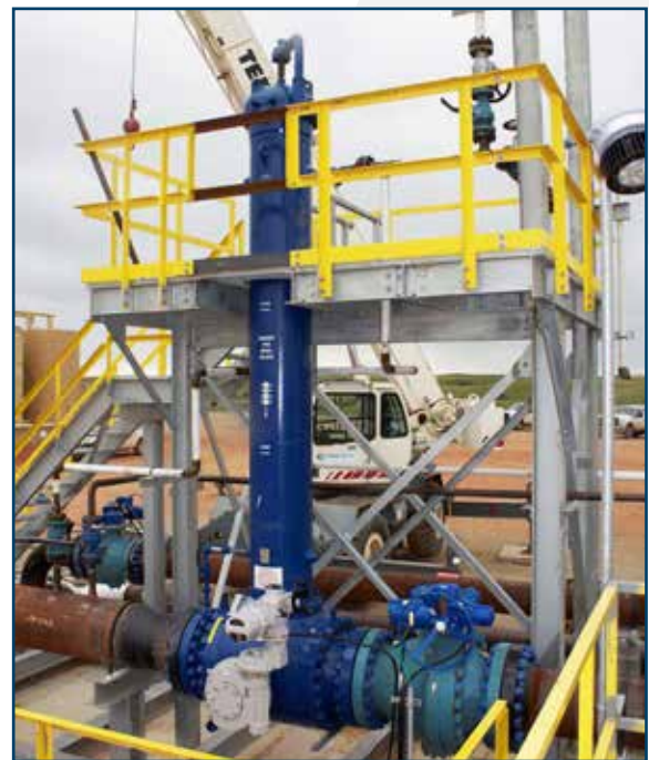
North Dakota, USA 16 inch 600 ASME, seven pig capacity. Electrically actuated.
