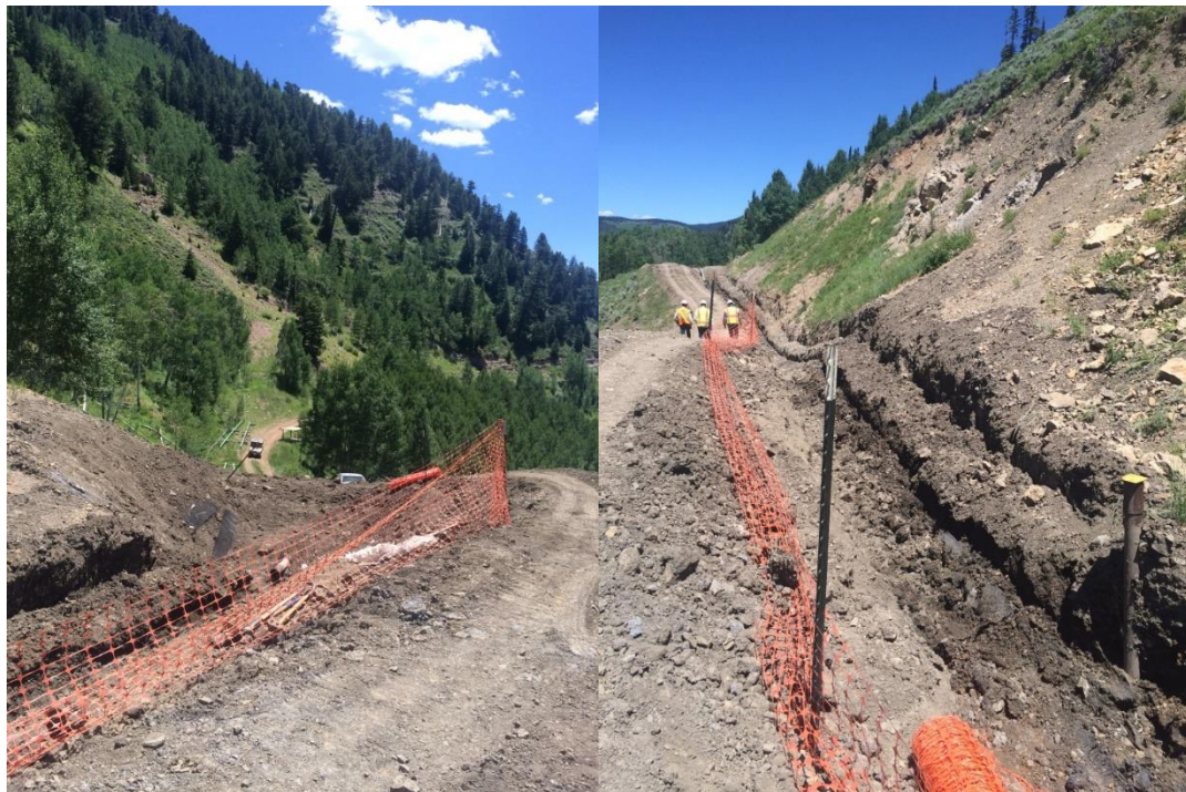
Figure 4: Examples of Terrain Where Circumferential SCC was Found.
