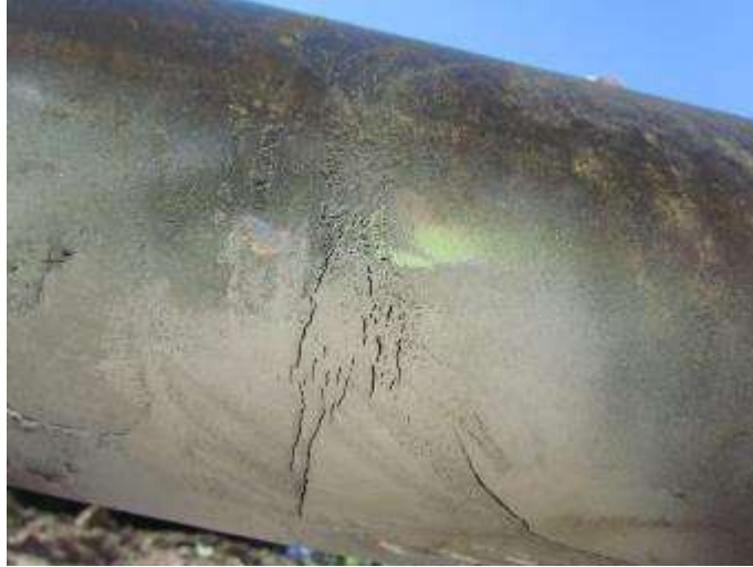
Figure 1: Circumferential Stress Corrosion Cracking (C-SCC) in a Natural Gas Pipeline
