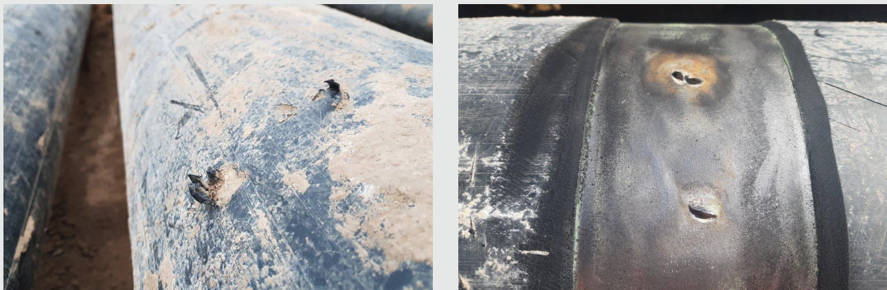
Figure 8: Coating holiday and underlying pipe wall anomaly (position +51 m in Figure 7)
