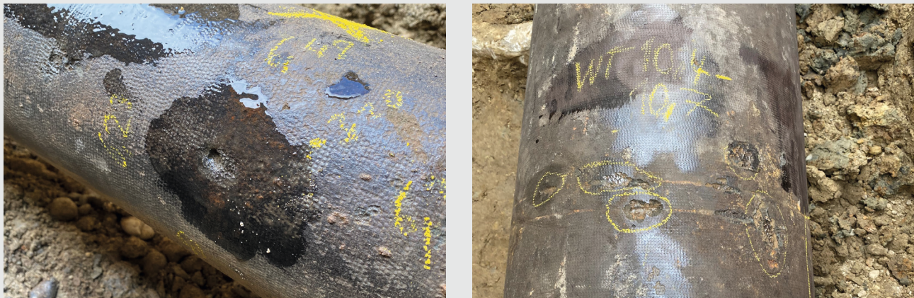
Figure 10: Two detected defects in the town of Grenchen, Switzerland
