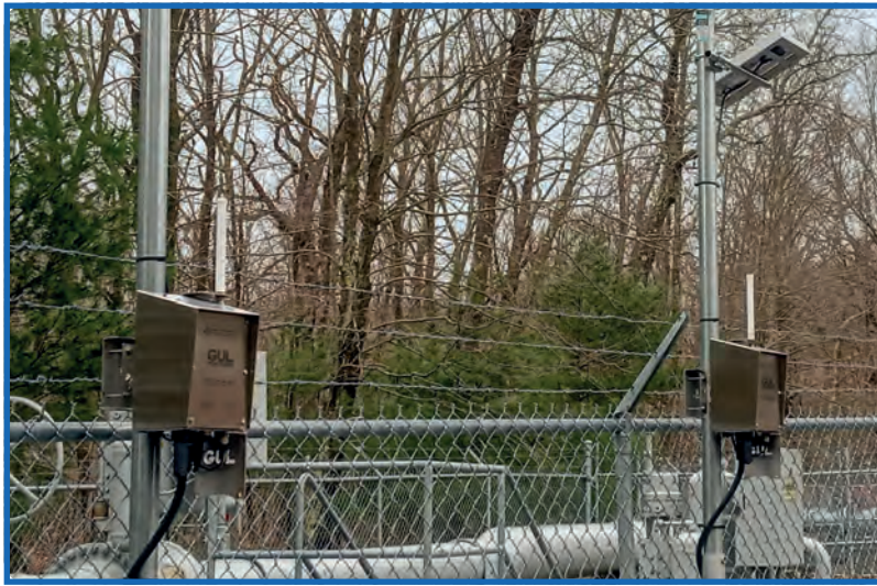
FCUs – solar-powered, connected to sensors on buried pipelines
