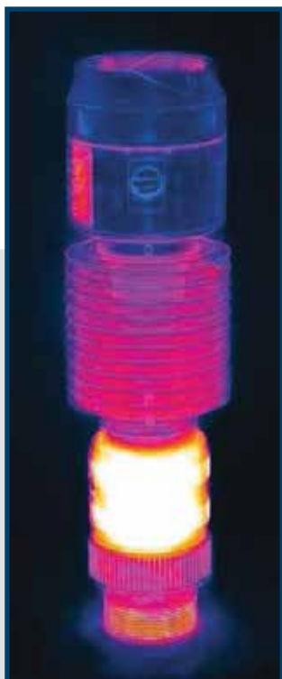
High Temperature Switch (Thermal Image)
