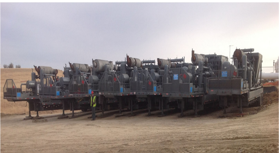
Seven units providing temporary compression during station outage
