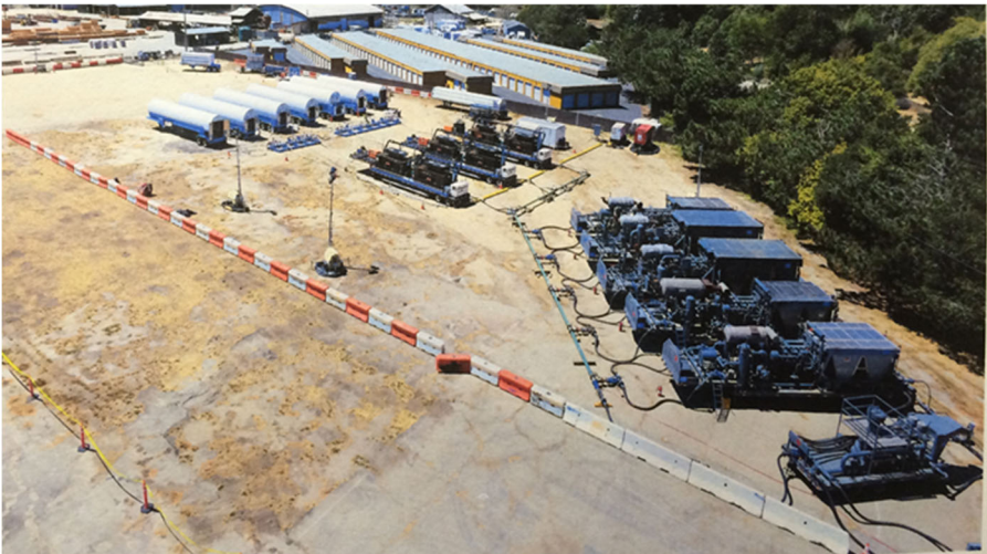
Compressors transferring vaporized LNG to supply pipeline
