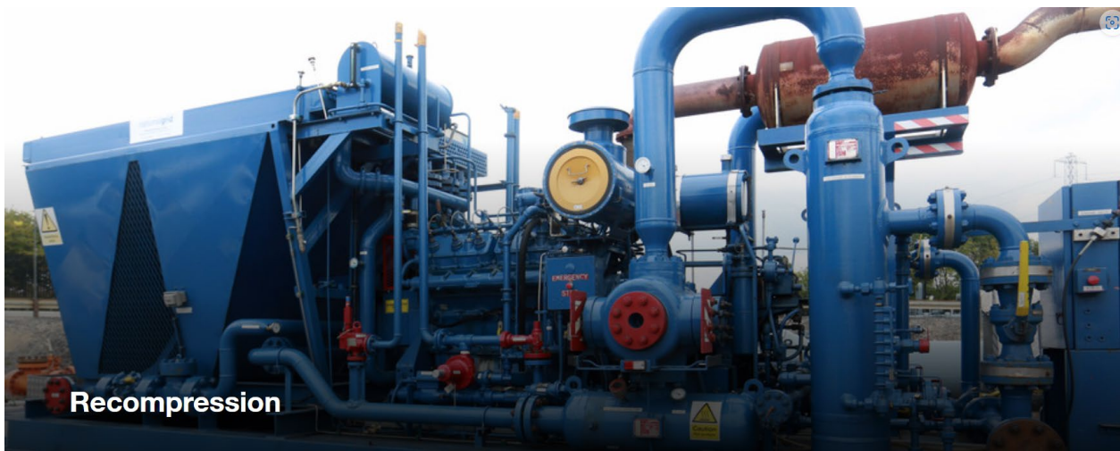
National Gas Recompression Unit (2) .
