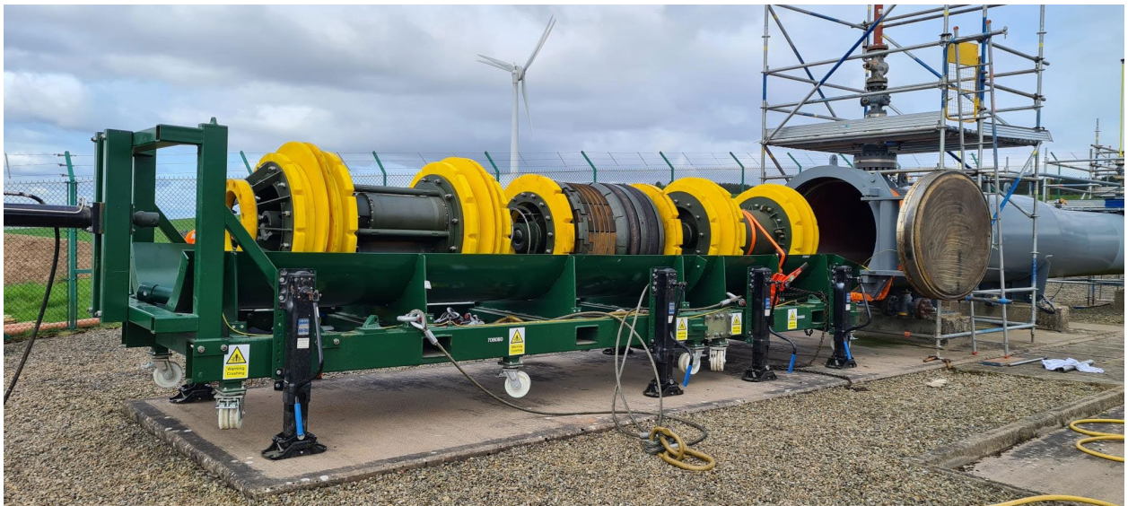
48" Remote Tecno Plug on Loading Tray at the Lochside Multi-Junction
