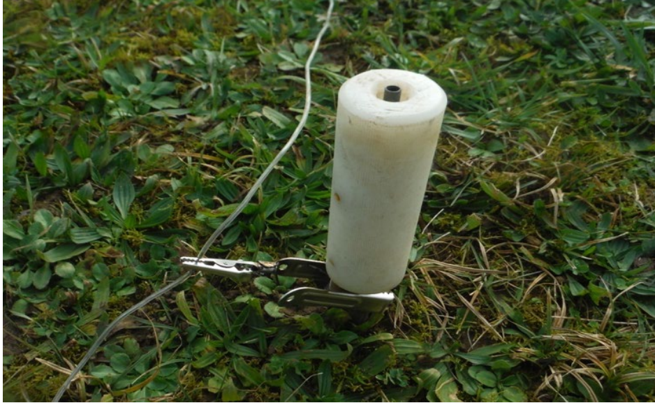
FIGURE 6. Earthing spike connected to the automatic timer
