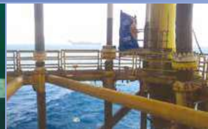
MECHANICAL DAMAGE, DENT, CRACK ...
