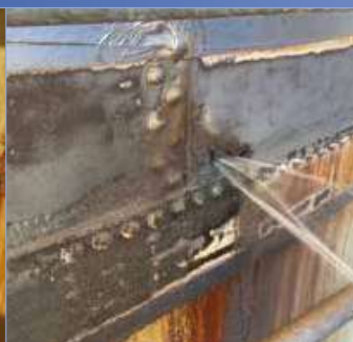
THROUGH WALL DEFECT, LEAK, HOLE
