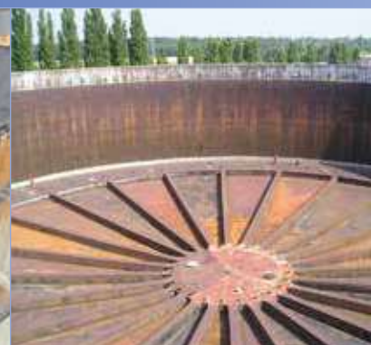
MECHANICAL DAMAGE, DENT, CRACK ...
