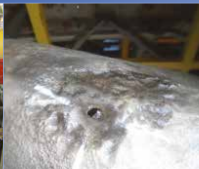
THROUGH WALL DEFECT, LEAK, HOLE
