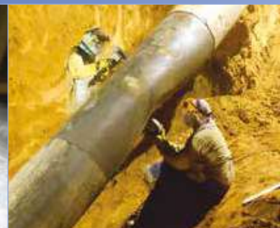
MECHANICAL DAMAGE, DENT, CRACK, SABOTAGE ...
